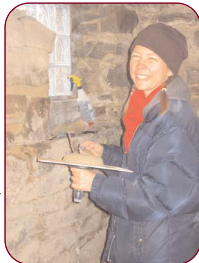
Laura Bidwa puts her skills to work at our March Masonry Repair Workshop.
